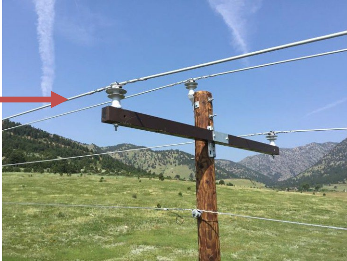
Three-phase covered conductor. (Blue Mountain 2)
